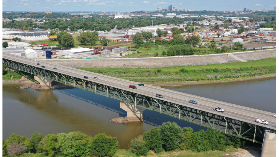
The 18th Street Bridge, built in 1959, is nearing the end of its service life.
